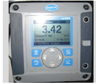
Controller (above left) indicating turbidity being about average for the test.
